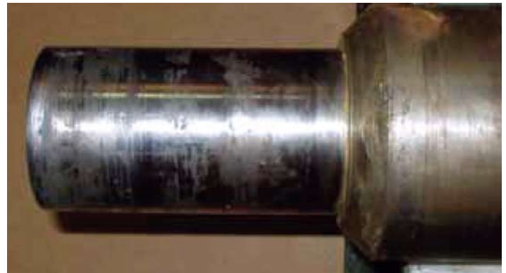
➔ The shaft is worn from an improper fit which creates contamination that could lead to early failure.
